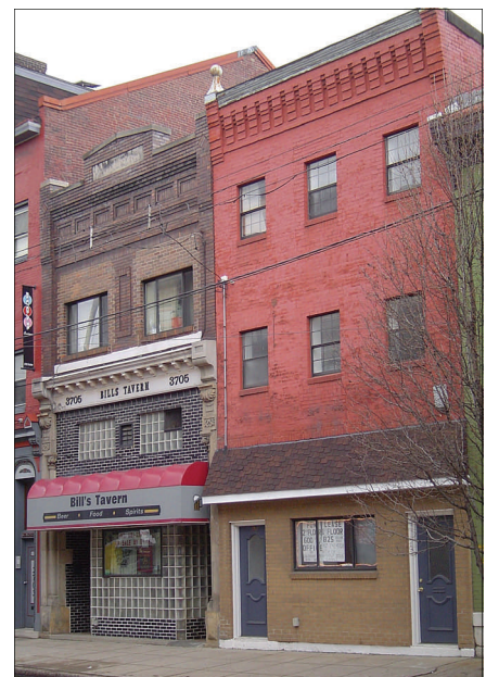
Figure 6. Inappropriate remodeling: closing up storefronts and windows, covering transom windows
